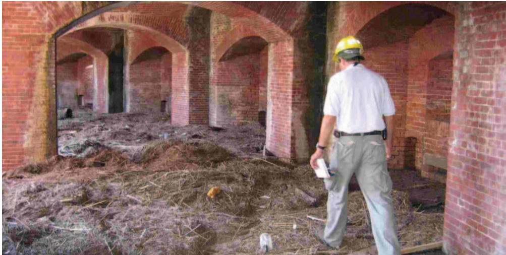
An NPS official surveys damage to Fort Massachusetts caused by Hurricane Katrina in 2005.
