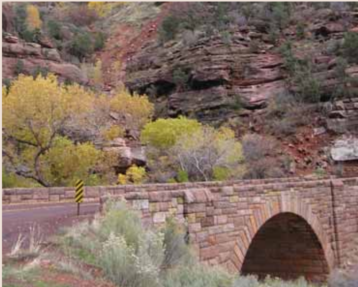
The multi-colored stone used to build the Pine Creek Bridge captures all the colors of the natural surroundings.
