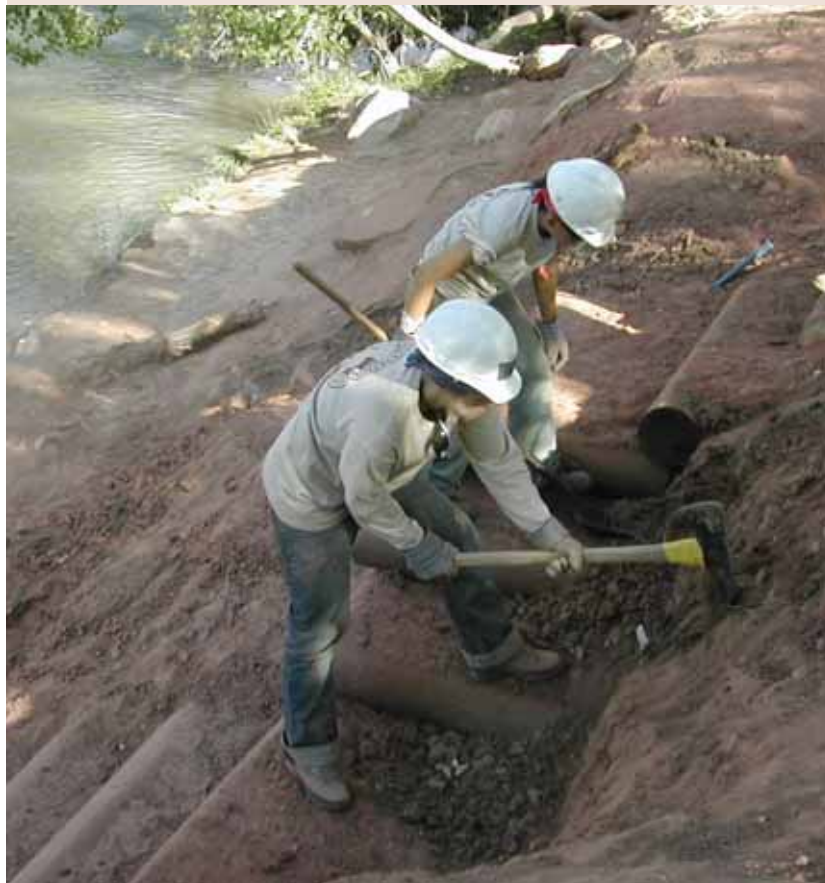
In 2004, 165 volunteers contributed 8,255 hours to various resource projects, a contribution valued at more than $115,000.
