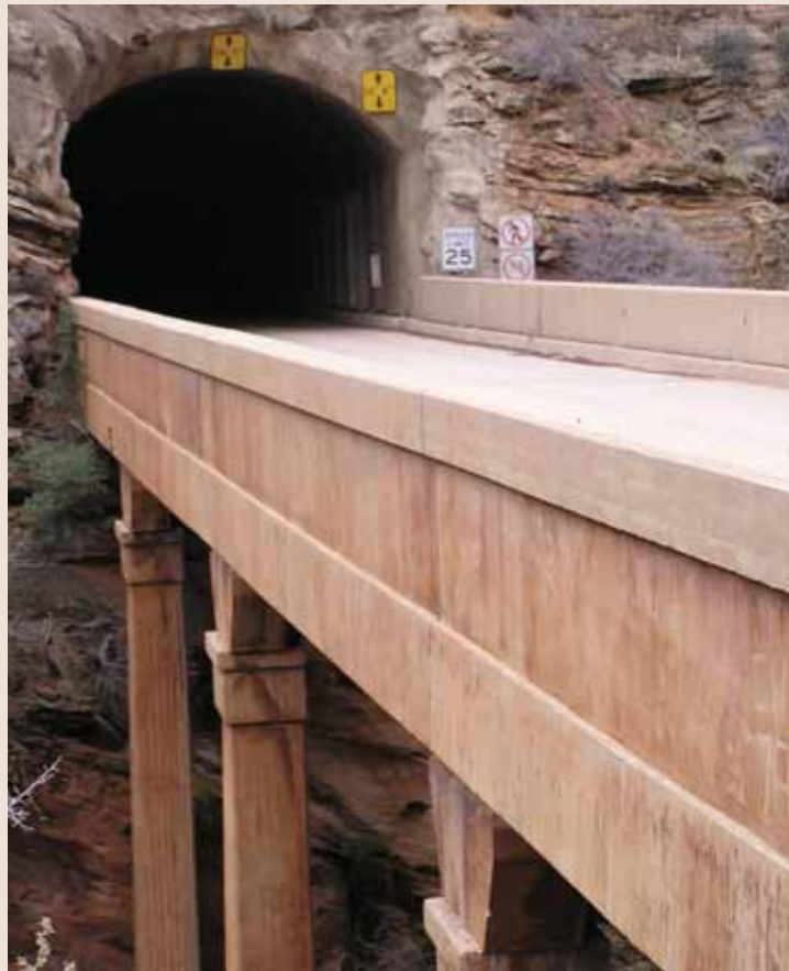
The Zion/Mount Carmel Road features a 5,613-foot long tunnel that was drilled through solid sandstone.
