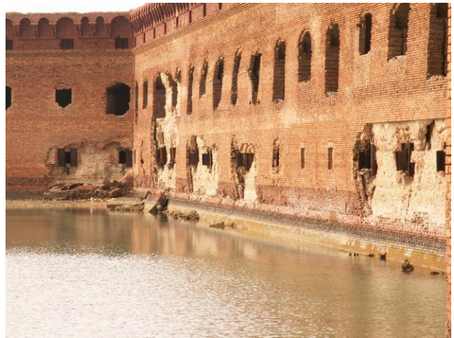
Crumbling masonry at Fort Jefferson. © John Adornato III/NPCA
