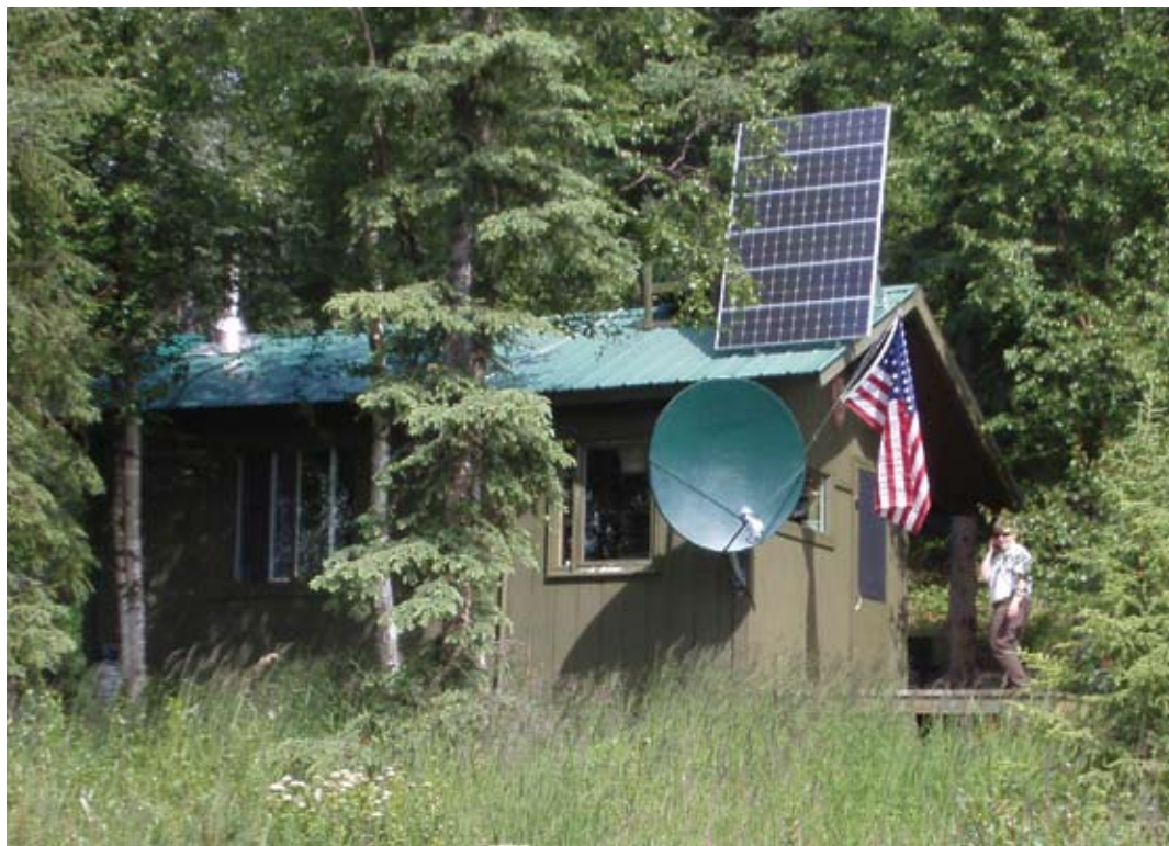
Solar panels at remote ranger stations, including those at the Telaquana Lake ranger station pictured here, help the park save money and lessen impacts on the environment.
