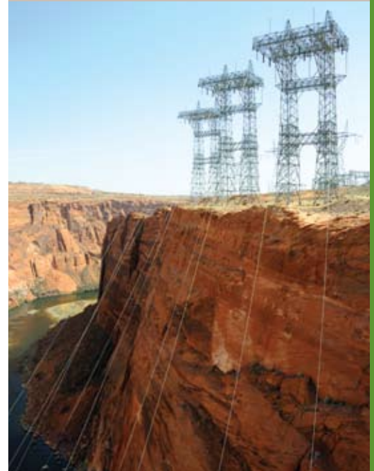
Above: Power transmission lines at Glen Canyon Dam. ©Gary Whitton.
