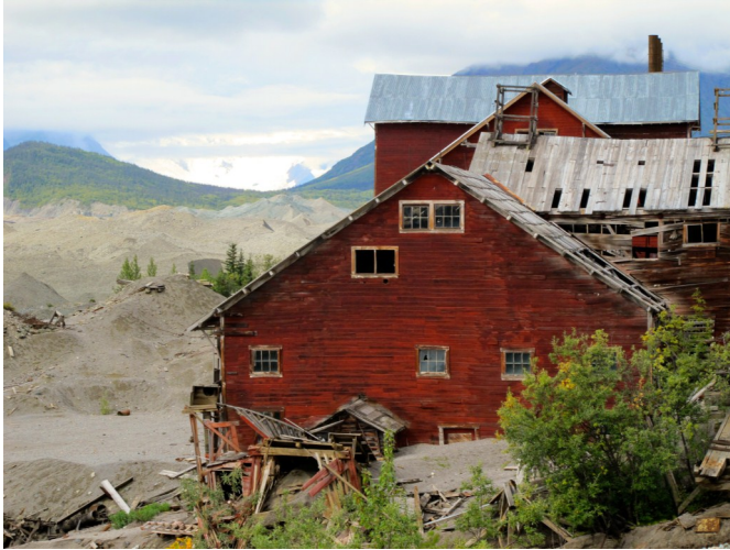
Kennecott Mill Complex, Wrangell-St. Elias National Park and Preserve. Many of the structures in this complex had been vandalized and were severely deteriorated when NPS gained ownership in 1998. The park is currently working to stabilize and/or rehabilitate some of the structures in order to interpret the history of this National Historic Landmark. Other structures will receive no treatment. Credit: Joy Stein/Shutterstock.
