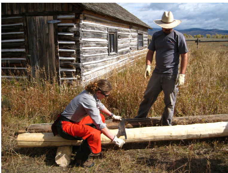
A National Park Service staff person demonstrating historic construction methods to a HistoriCorps volunteer during the Chambers Residence rehabilitation. Credit: HistoriCorps.
