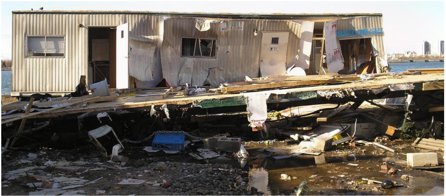
Park facilities damaged on Ellis Island National Monument. Photo by NPS/Bauer
