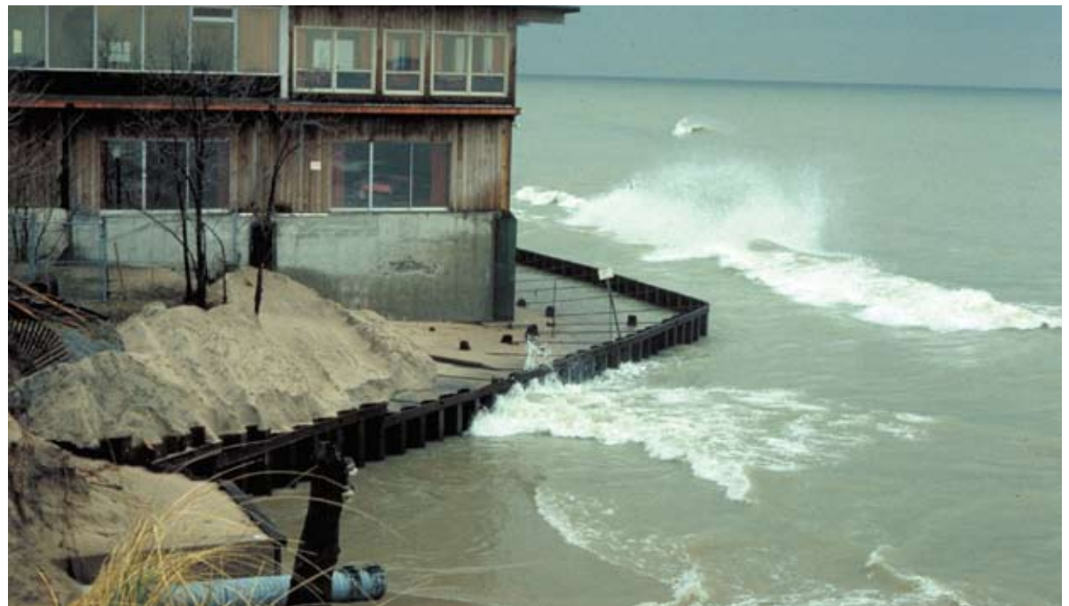
ABOVE: Shoreline erosion - Red Lantern Restaurant, Lake Michigan, Indiana. NPS
