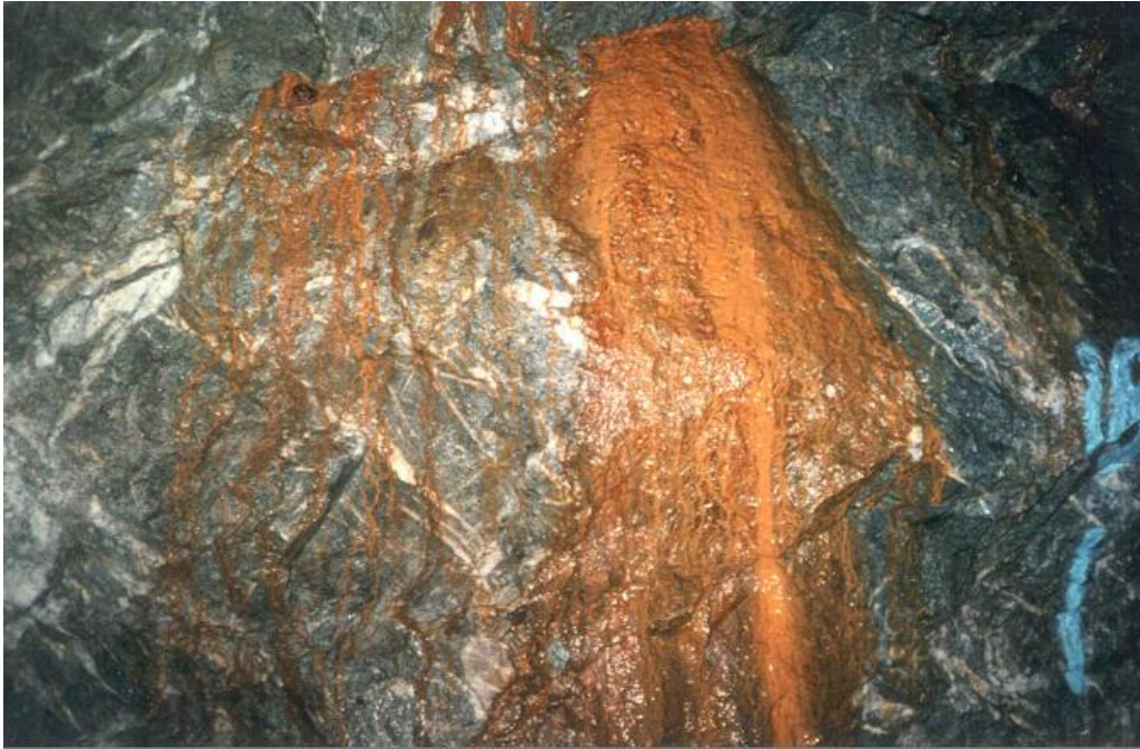
Figure 1: Acid Mine drainage seeping through a rock wall at Kensington Mine, near Juneau AK
