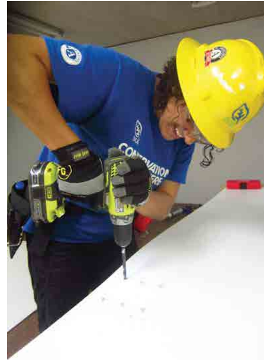
A Student Conservation Association crew member works to rehabilitate a building at Camp Ken-Etiwapec in New Jersey, a former Boy Scout camp in the park. The camp will house youth corps crews engaged in future historic preservation training programs and projects in and around Delaware Water Gap National Recreation Area. The work was part of the Hands-On Preservation Experience (HOPE) Crew partnership between the National Trust for Historic Preservation and The Corps Network. It was funded by the National Park Service, and supervised by Philadelphia preservation carpenter, Mathew Grubel. © Steve Cimbalik
